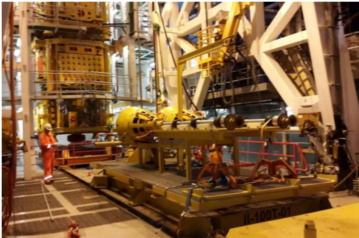
PCH Skid with Stack in garage
