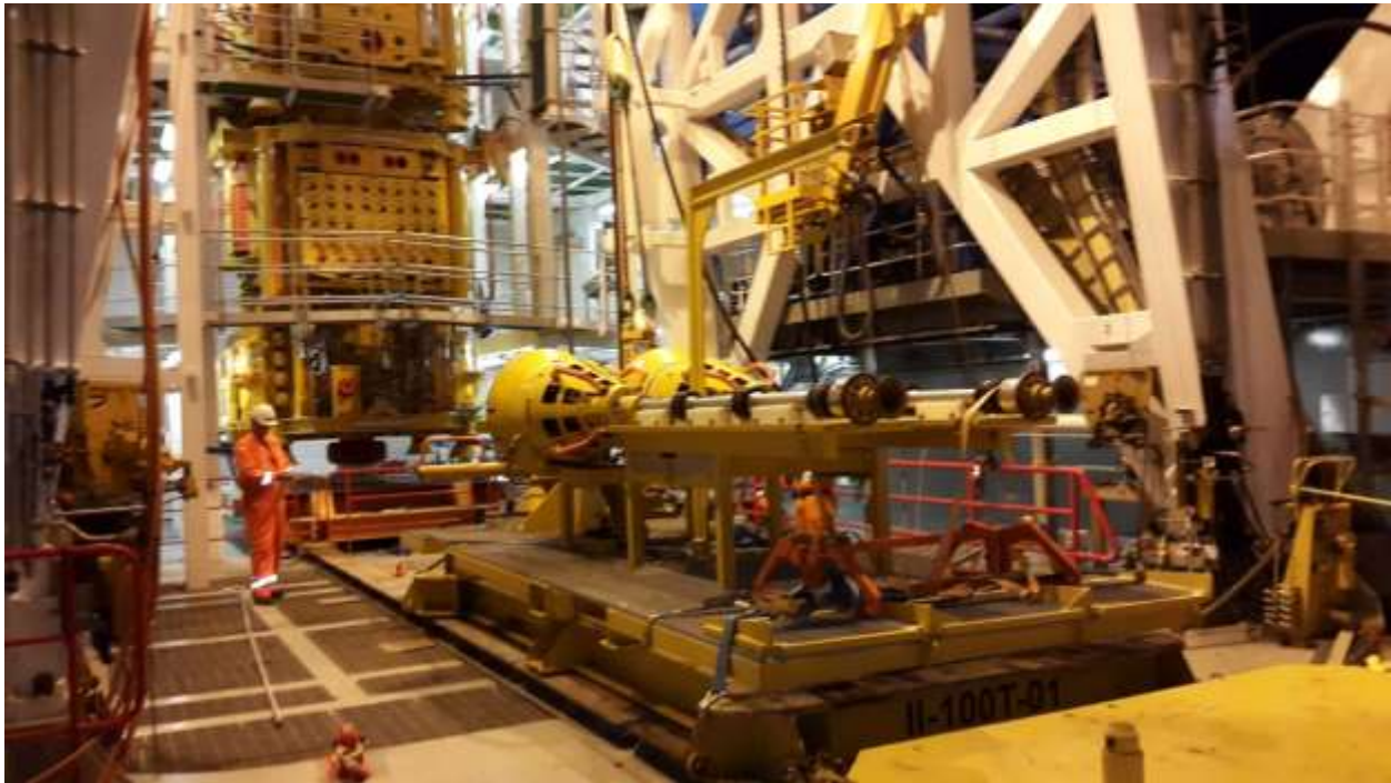
TFMC Well Control Package in garage with Pressure Control Heads on pallet over the moonpool onboard LWIV Island Performer GoM 2015
